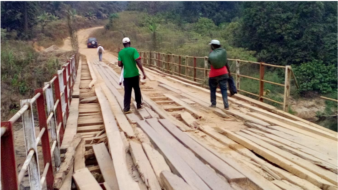
Picture 2. This decayed bridge deck illustrates the constraints that hamper mobility and, therefore, face-to-face meetings. This photography has been taken in Mabombe (district of Loum) in 2016.
